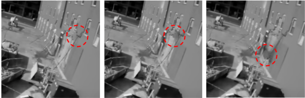
43. Approximately 56 seconds before the catastrophic collapse more bricks crumbled out of the bottom of the wall, stripping away even more of the wall's structural support.
